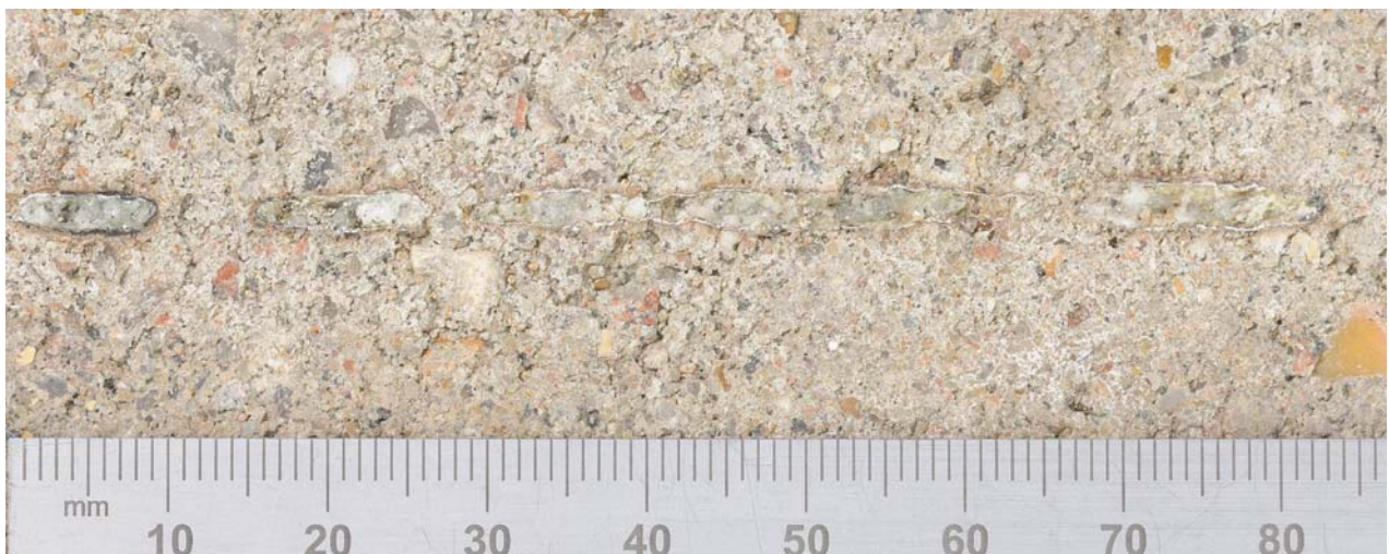
Figure 12 Effect on the concrete surface after removal of the steel.
