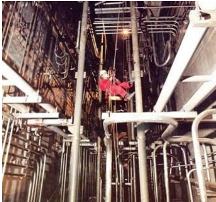
Figure 1 – Complex process cave (photo taken during commissioning)
