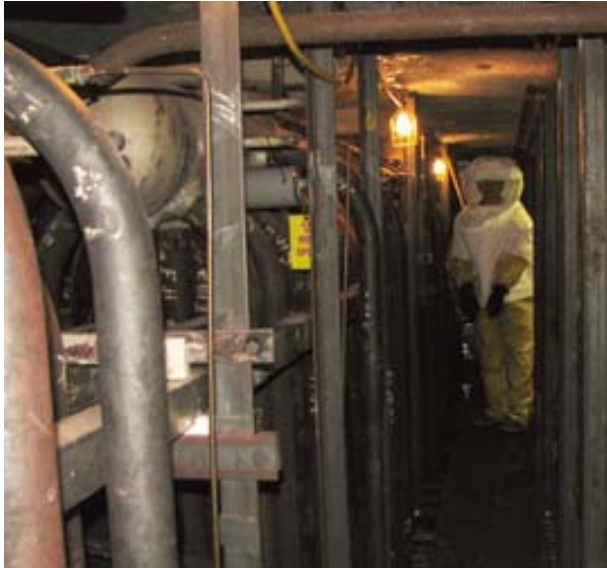
Upper feeder cabinet (UFC)
