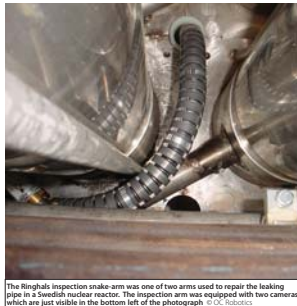
The Ringhals inspection snake-arm was one of two arms used to repair the leaking pipe in a Swedish nuclear reactor. The inspection arm was equipped with two cameras which are just visible in the bottom left of the photograph © OC Robotics
