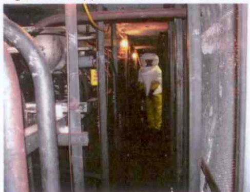
Figure V.3: Upper Feeder Cabinet
