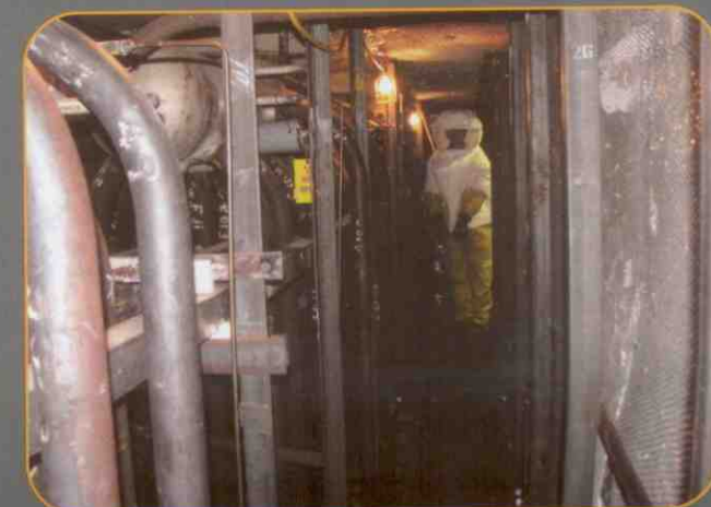
Upper Feeder Cabinet
