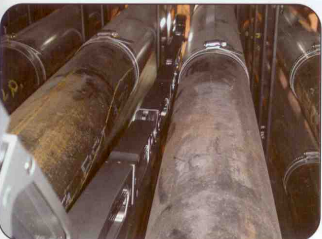
SAFIRE with arm deployed below the walkway (in mock up)
